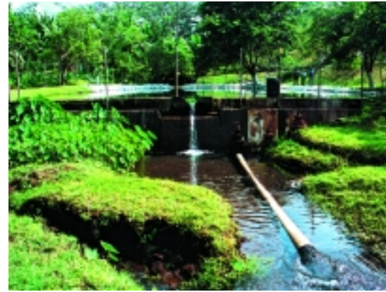
Decentral water purification plant.
